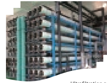
Ultrafiltration and reverse osmosis equipment
