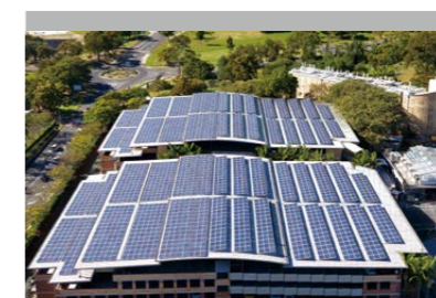
Commercial PV system
